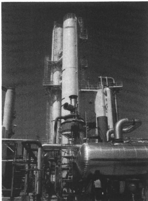
Figure 17. A Modern Cryogenic Air Separation Plant. (Courtesy of PRAXAIR Technology, Inc.)
